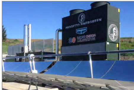
The solar concentrators; behind them, the cooling tower
