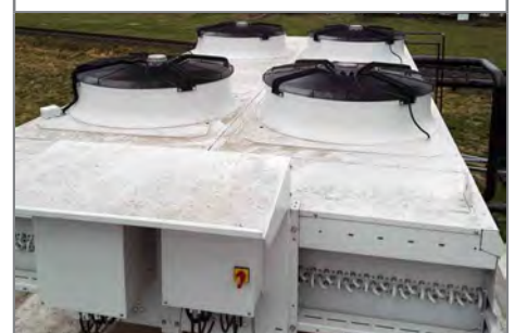
A detail of the dry cooler placed on the roof
