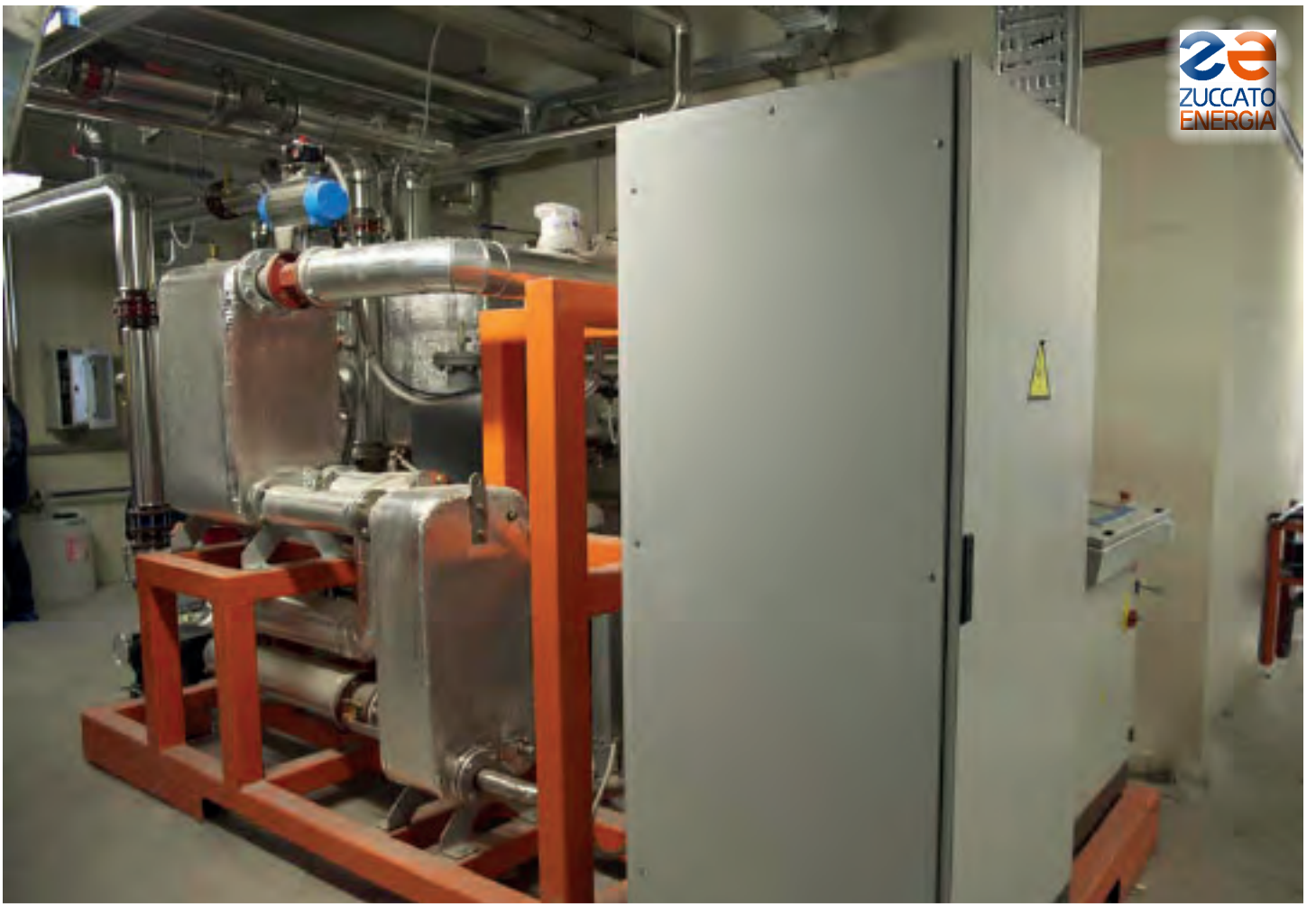
South Tyrol 03 / Meran: The ZE-50-ULH low-temperature ORC module at the customer's site, viewed from the side.
