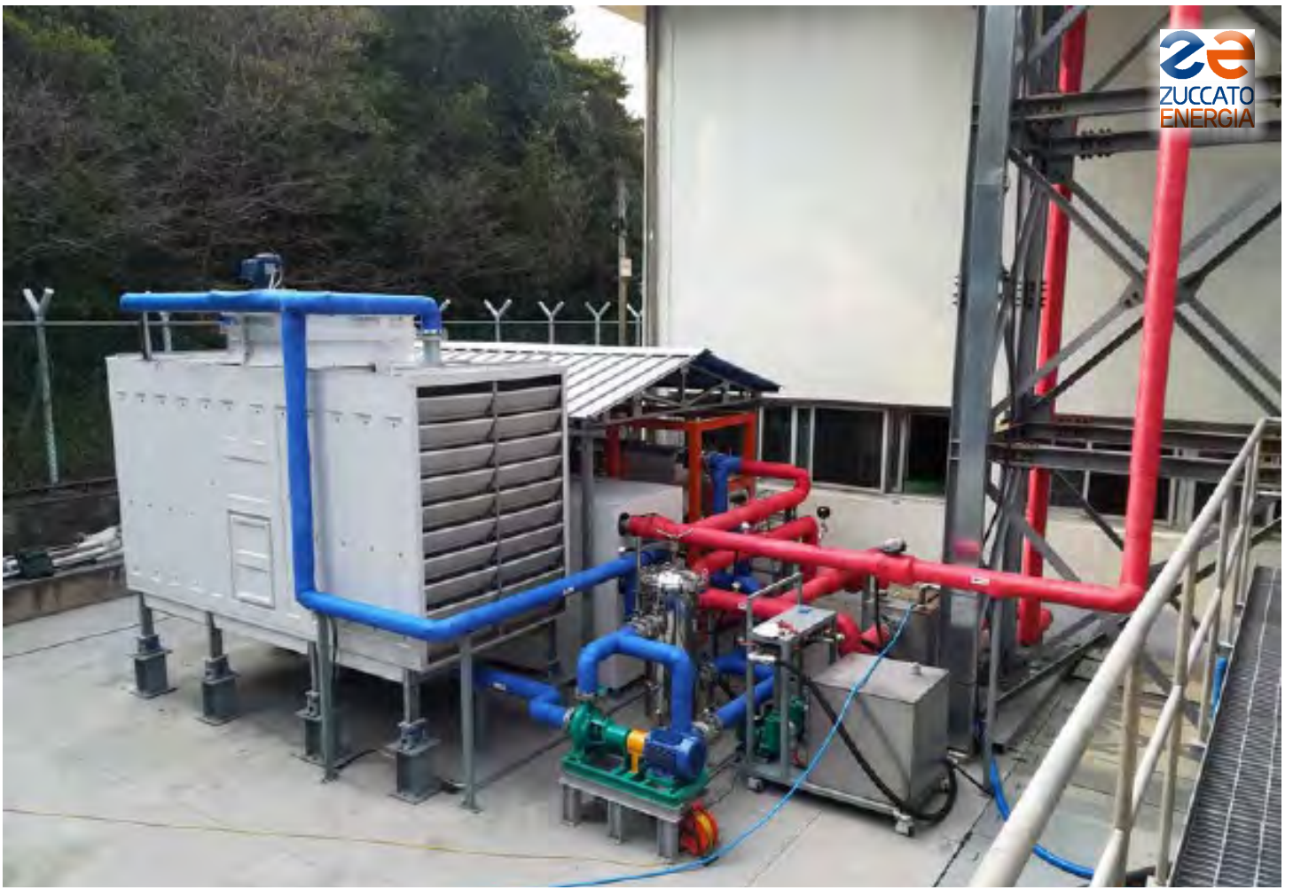
Korea 01 : The cooling tower and the awning hosting the ZE-40-ULH organic Rankine cycle power generation module
