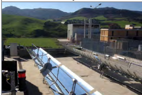
An overview of the solar concentrators area
