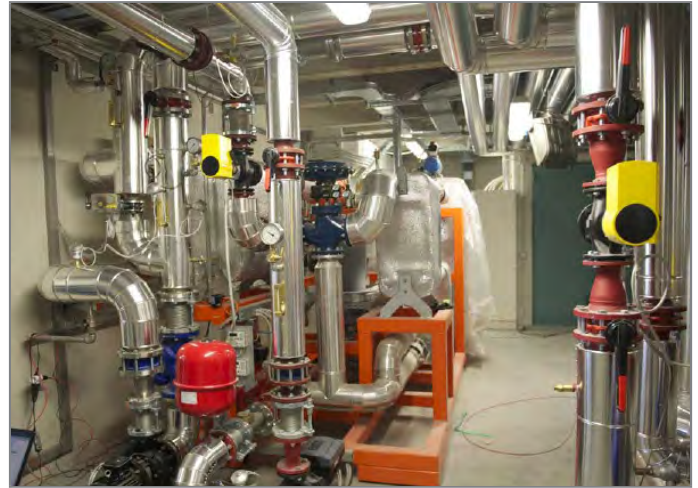
The skid in place seen from the side of the hydraulic connections
