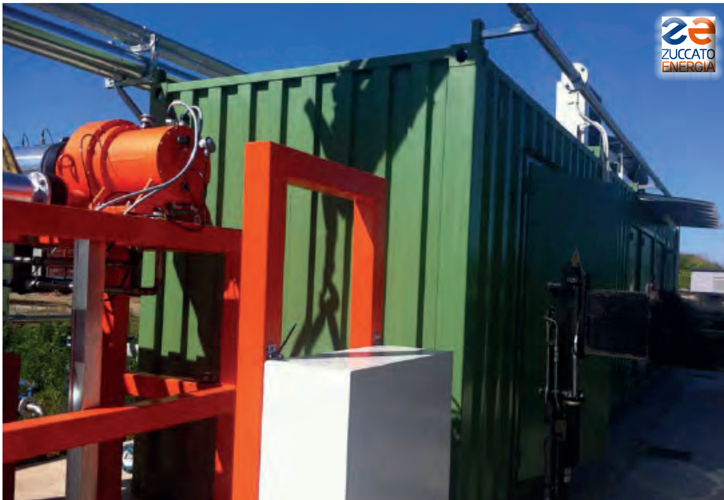
Veneto 02 / Padoua: The ORC module (orange) with its terminal block (white) and the containerized control room (green).
