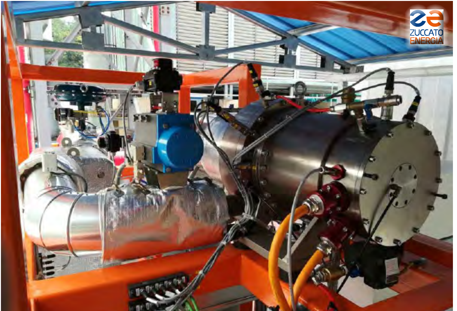
Korea 01 : A detail of the ORC skid - the steel cylinder in the middle is the turbogenerator
