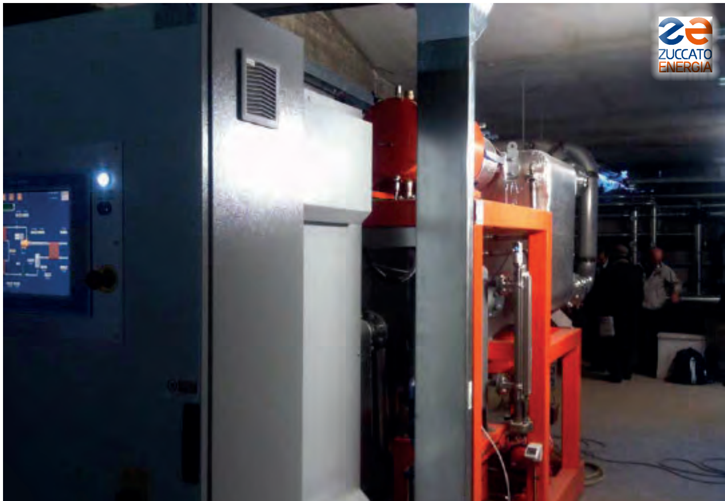
Lazio 01 / Roma: ORC module ZE-50-ULH in its underground room located under one of the movie theaters.
