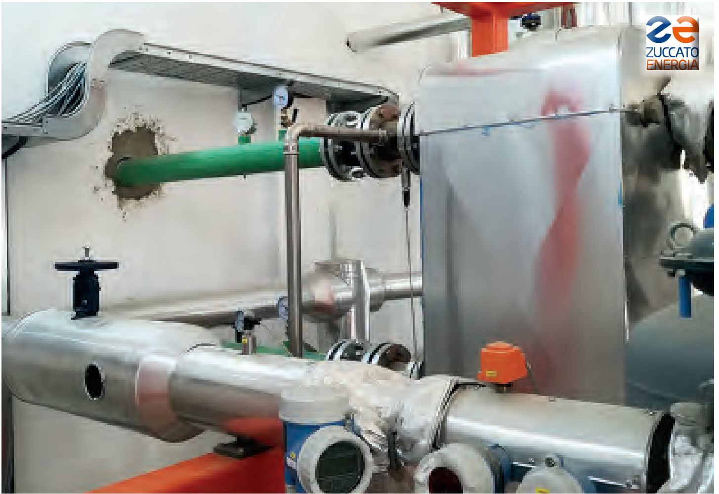
Tunisia 01 : The heat exchangers. This is the first plant by ZE using live saturated steam as a vector fluid.
