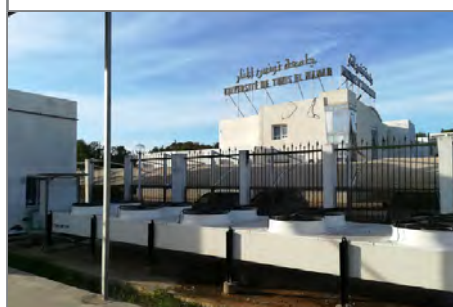
The dry coolers with the main campus building in the background
