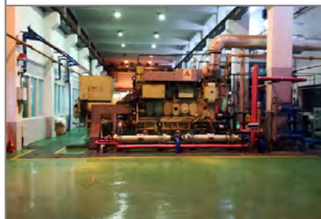
The large diesel genset from which waste heat is recovered
