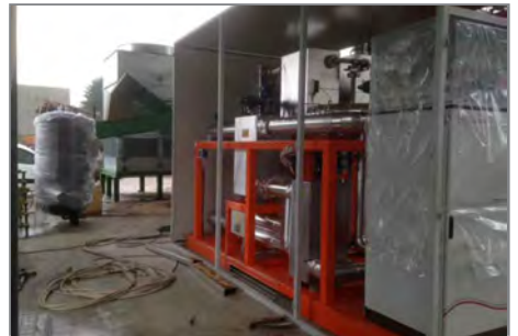
The skid during installation in the soundproof enclosure.
