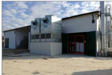
The boiler building hosting the ORCs and the boiler.
