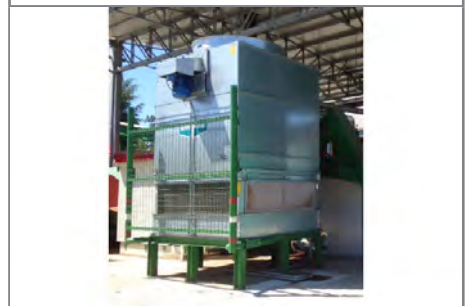
The cooling tower: some of the waste heat is used to dry the wood chips.
