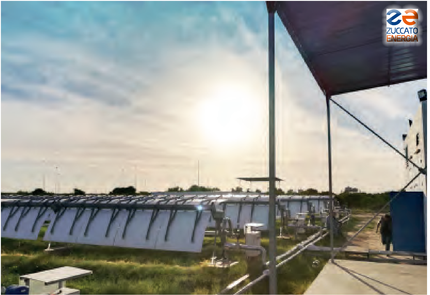
Tunisia 01 : The solar field at sunset, taken from the canopy adjacent to the building housing the skid.
