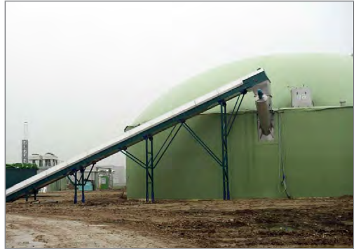
The slurry loading auger
