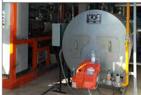
The biogas boiler (R) and the ORC module skid (L)
