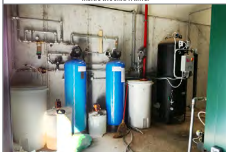
The water treatment system feeding the evaporative cooling tower.
