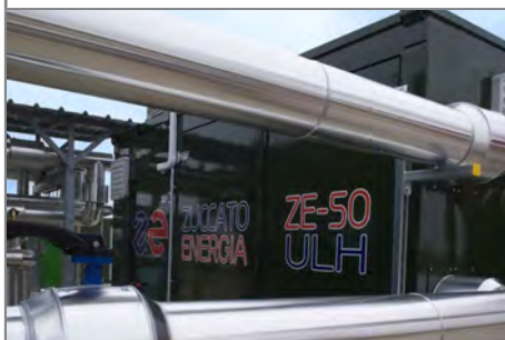
The ORC module from the control panel side
