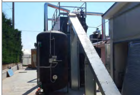
The wood chips loading screw which brings fuel to the boiler
