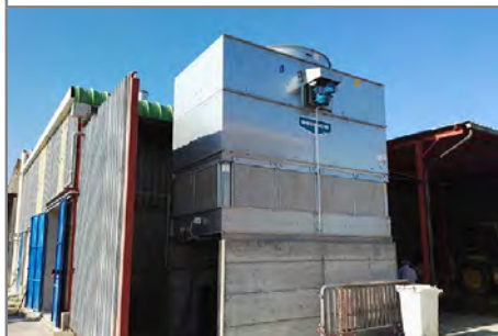
The cooling tower
