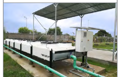
The dry coolers from the opposite side
