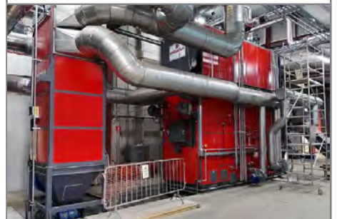
The boiler seen from the flue gas processing side
