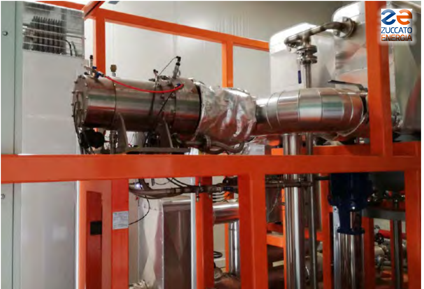
Lombardia 03 / Brescia: A detail of the ORC skid - the steel cylinder in the middle is the turbogenerator
