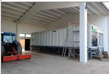
The biomass loading hopper.
