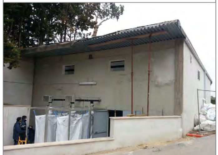
The gasifier room with ash discharge in the foreground
