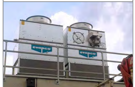
The cooling towers for the condensing stage.
