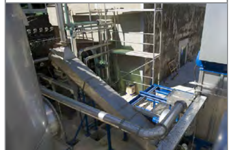
General view of the fuel loading auger
