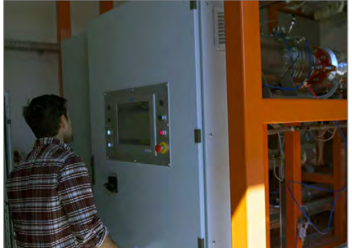
The ORC skid control panel
