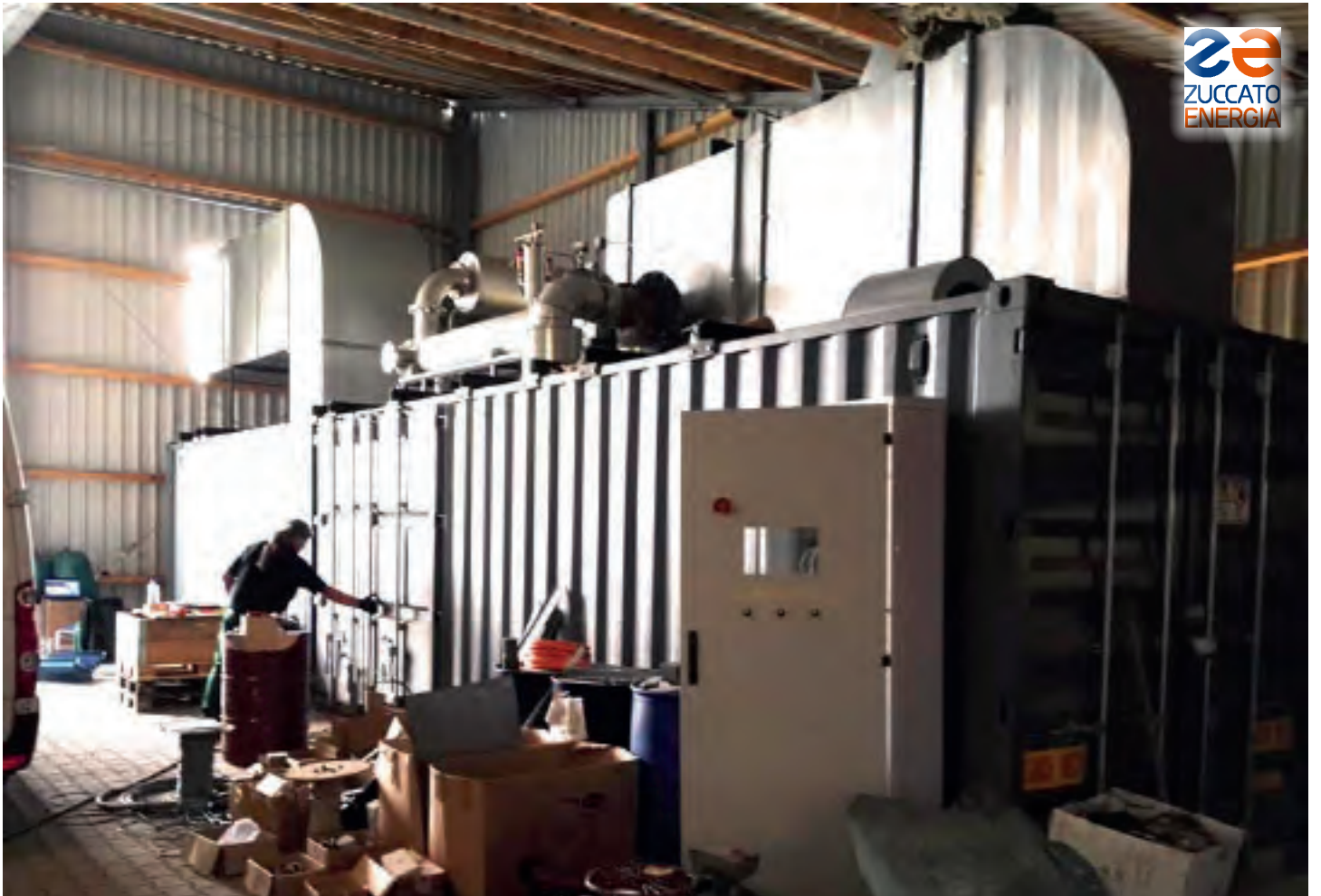
Germania 02 / Bassa Sassonia: The container hosting the biogas-fueled MAN gaset
