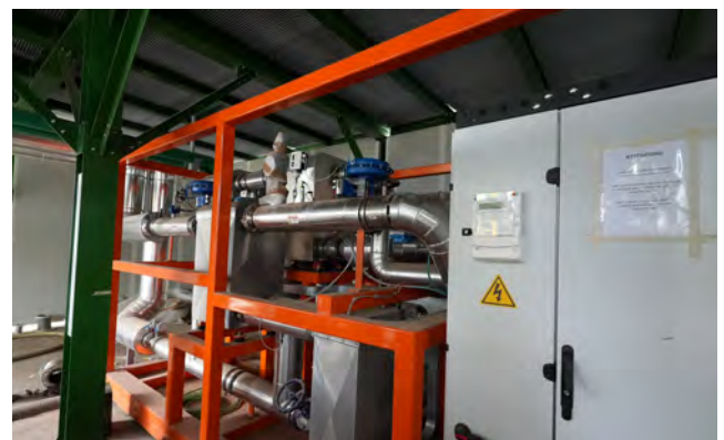
ORC system's electrical cabinet
