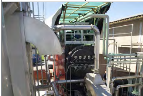
A detail of the loading auger and burner
