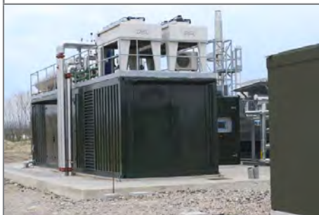
The container housing the biogas engine
