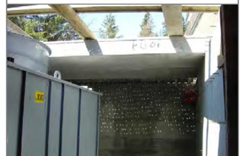
The cooling tower, housed in an underground room with a grid ceiling
