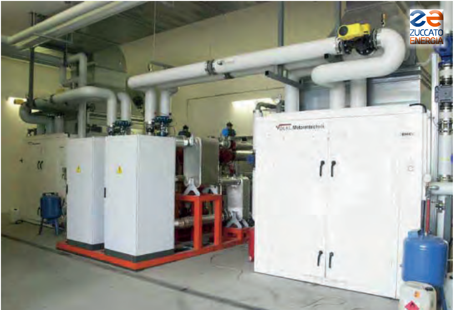
South Tyrol 04 / Bolzano: The complete installation with both modules, flanked by the motors whose heat it recovers.
