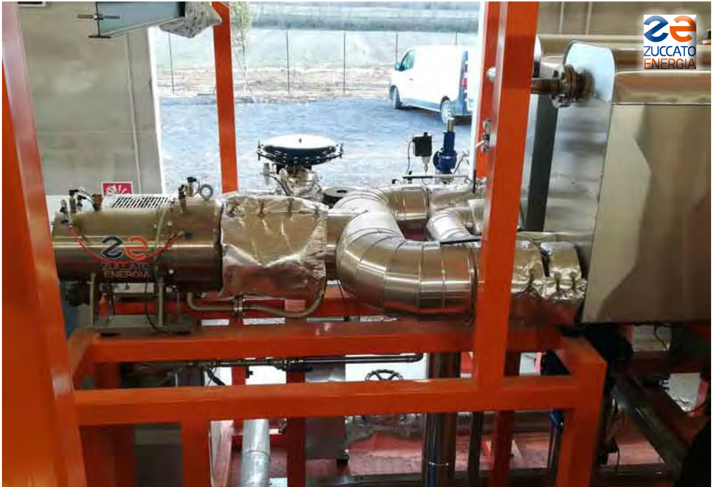
Umbria 01 / Perugia : A detail of one of the two ZE-100-LT ORC modules in their own room
