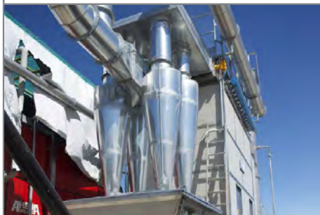
The flue gas treatment plant with the cover removed To show the filter cyclones
