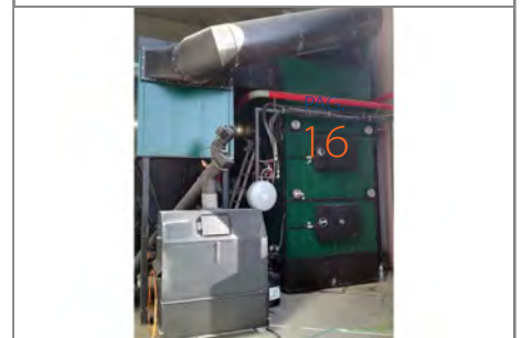
The boiler (R) and the ash filter (L).
