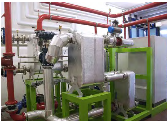
The ORC module at the headquarters
