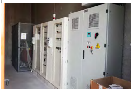
The mains grid interface panels.
