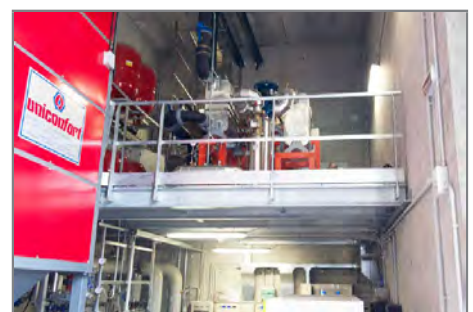
View of the mezzanine hosting the ZE-50-ULH system
