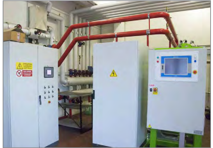
The plant control panels
