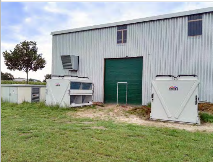
The entrance door and the dry coolers for the condensation stage
