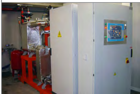
General view of the ORC ZE-40-ULH module from the switchboard side
