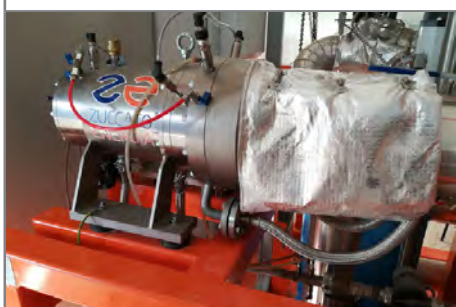
A detail of the plant's custom turbine
