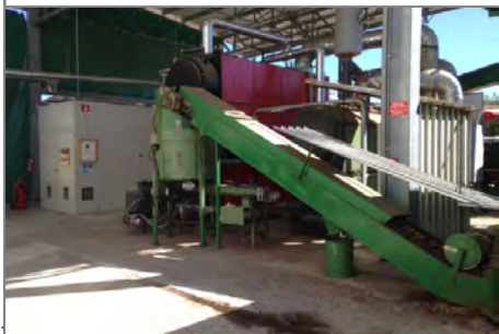
Detail of the wood chip conveyor to the boiler. On the bottom the skid.
