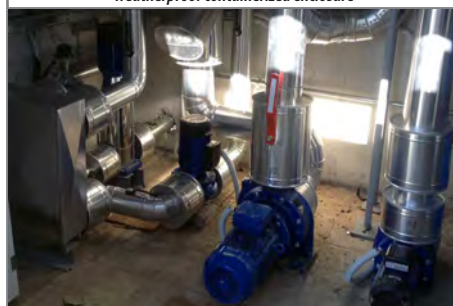
The pumps which manage the hybrid heating system
