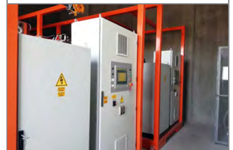
The control panels for the ORCs
