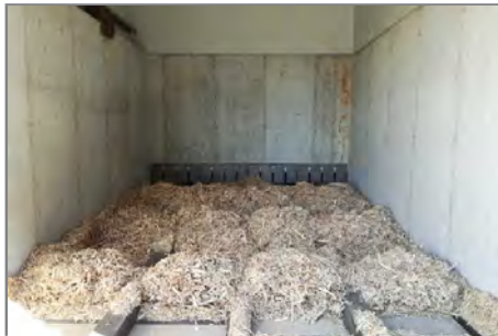
The biomass hopper, with a rake-style feeding system.
