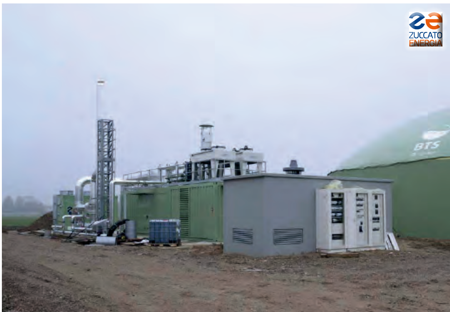
Lombardy 01 / Mantua: General view of fermenters, motors and the containerized ORC ZE-50-ULH module.
