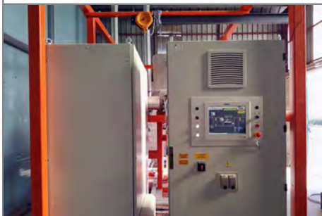
A detail of the ORC module control panel
