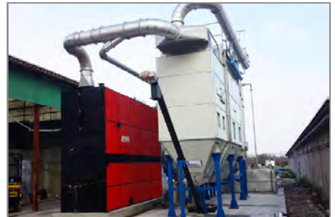
The boiler (left) and the flue gas treatment plant
