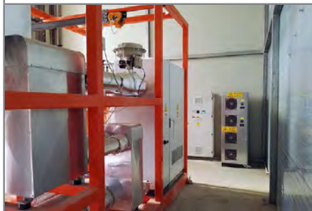
The ORC module; in background, the braking resistors cabinet
