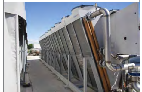
A detail of the dry cooler
