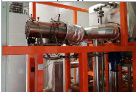
The turbogenerator (silver cylinder) inside the skid frame.
