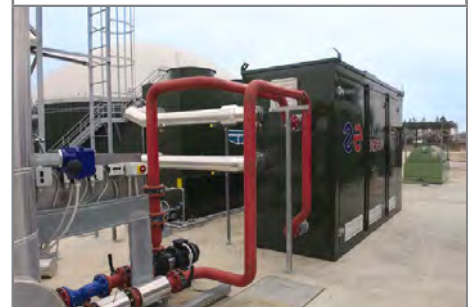
The ORC module from the control panel side
