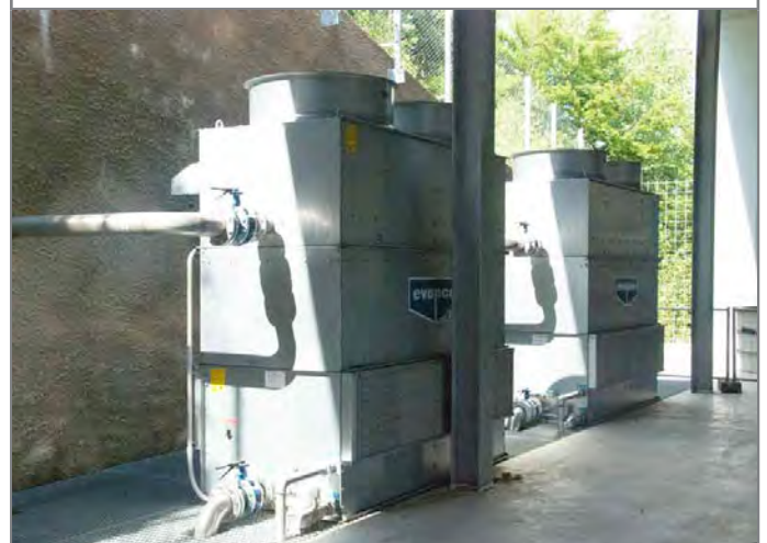
The cooling towers, located at the back of the building.
