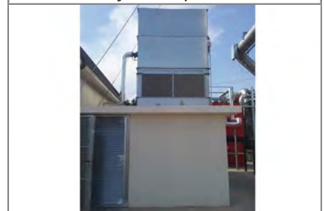
The cooling tower which dissipates the excess heat of the ORC condensation stage
