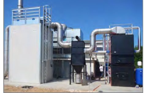
R to L: boiler, dust trap and and flue gas treatment system
