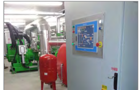
Interior view of the thermal power plant
