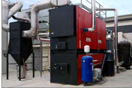
The 1300-kWT movable grate boiler, fueled by wooden chips.
