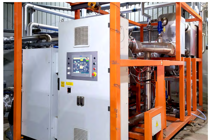
The ZE-105-CHP ORC seen from the control panel side
