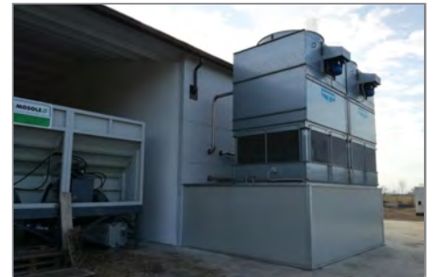
The evaporative cooling tower.
