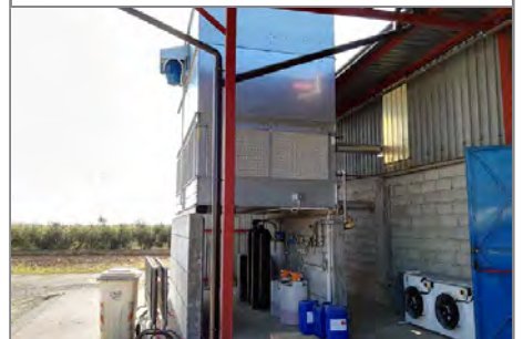
The tower base hosts the cooling water treatment system
