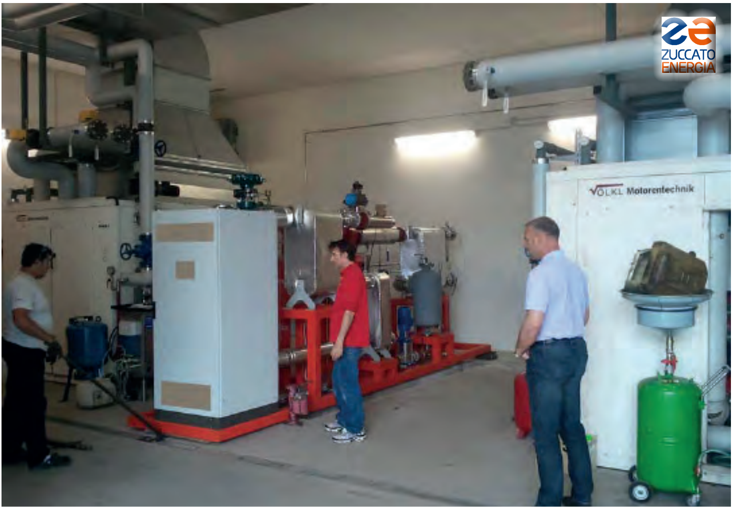
South Tyrol 04 / Bolzano: The first ORC ZE-50-ULH module during installation. Note the custom-made skid.
