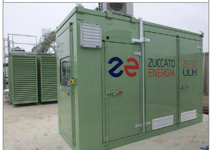
The right side of the containerized ORC module.
