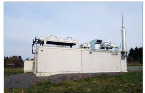
The east side of the prefab. On the roof, the dry cooler of the condensation stage.
