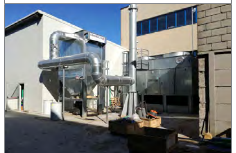
L to R: the bag filter for flue gases, the chimney and the cooling tower.
