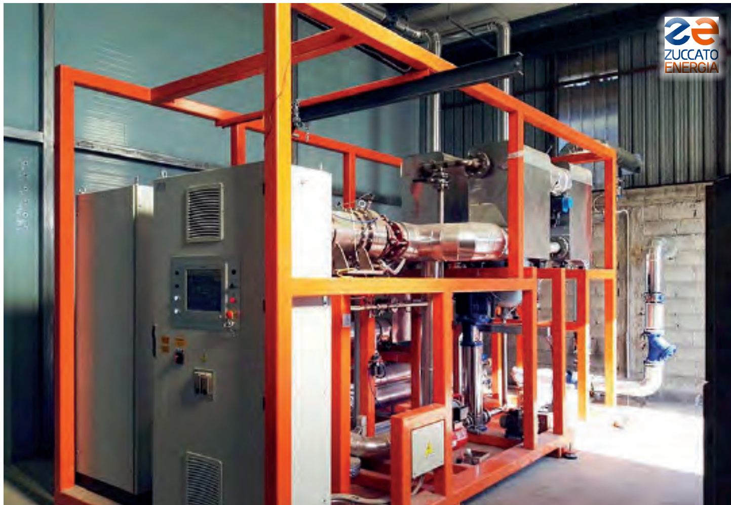
Calabria 01 / Cosenza : The ZE-175-LT ORC module in its place, seen from the control panel side
