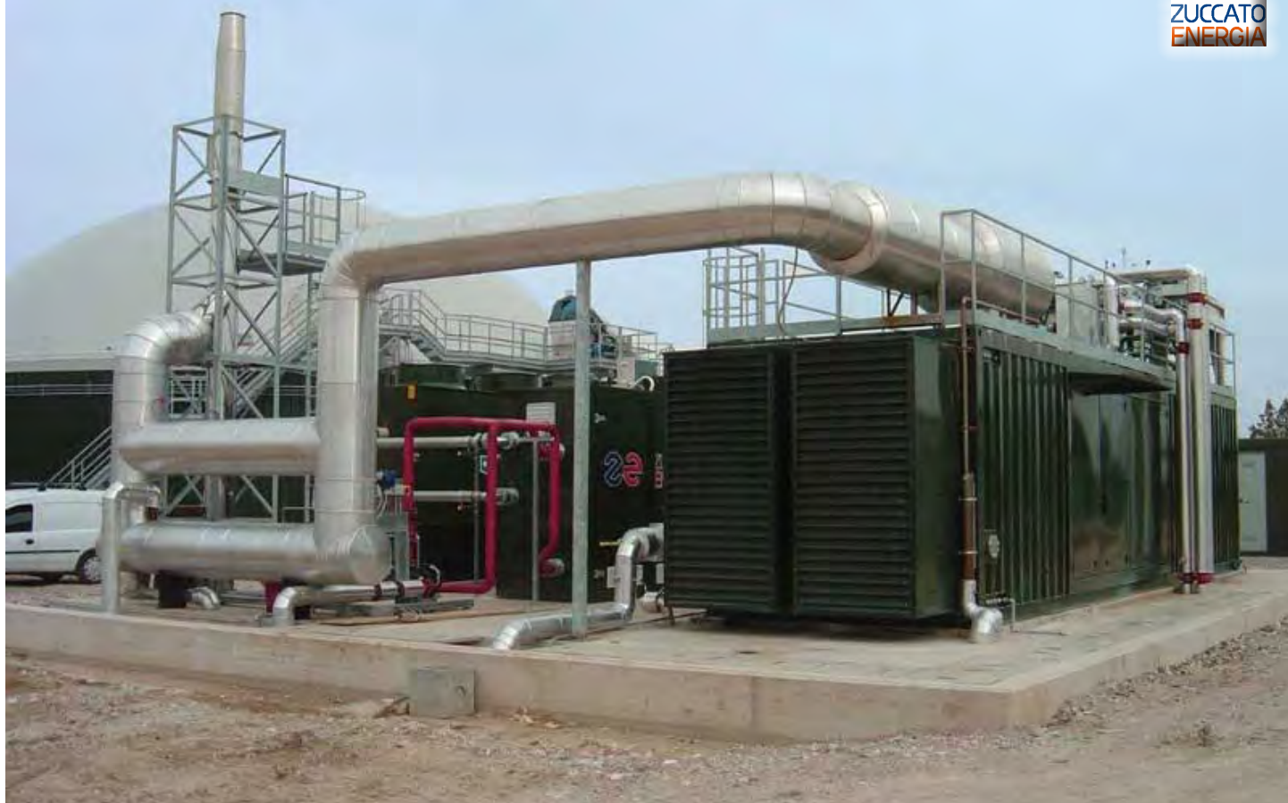
Veneto 01 / Venice: An overview of the entire facility from the rear side.
