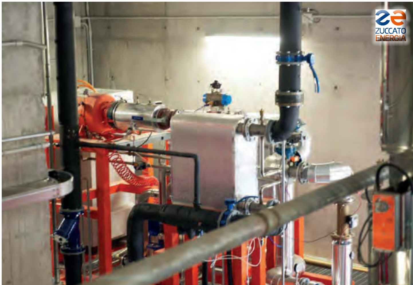
Veneto 03 / Venice The ORC ZE-50-ULH module on site at the customer's premises, seen from above.
