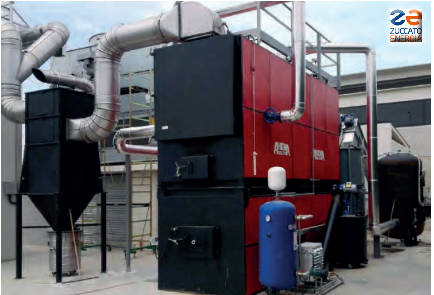
Sicilia 01 / Ragusa : The 1.3MWt moving grate boiler , fed with wood chips (fruit crate production waste)
