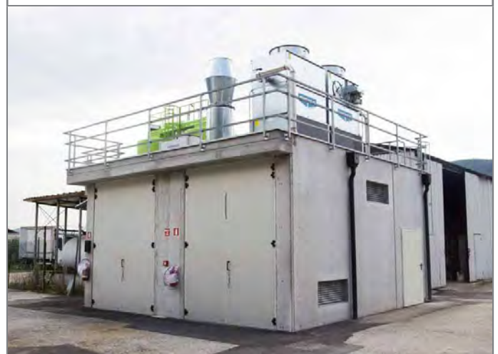
The structure that houses the skid
