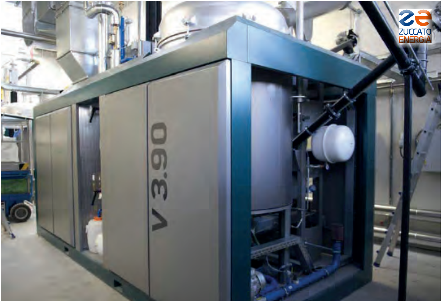
South Tyrol 03 / Meran: One of the gasifiers from which the ORC module recovers thermal waste.
