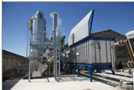
Fuel loading hopper and chimney
