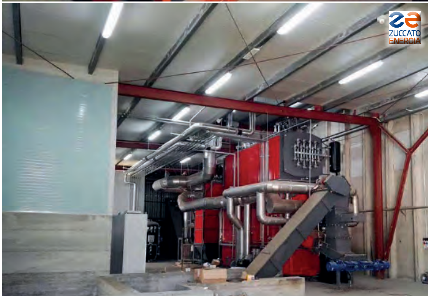
Calabria 01 / Cosenza : The boiler seen from the biomass loading side
