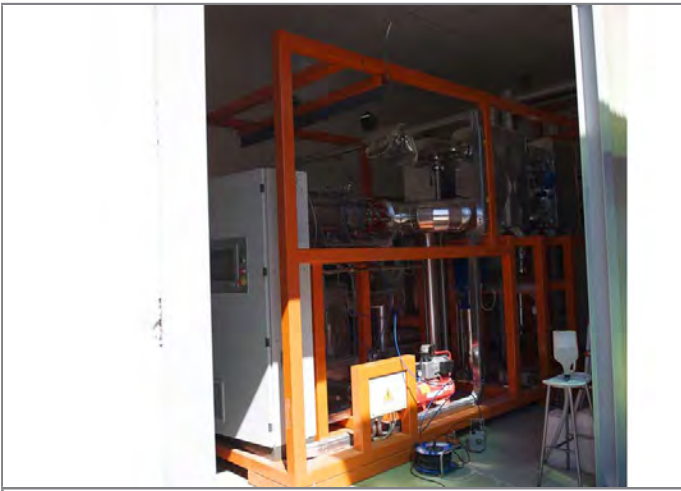
General view of the ZE-150-LT module in its shelter
