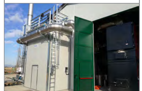
The flue gas treatment system and the boiler room
