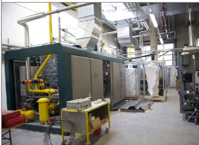
General view of Burkhardt gasifiers
