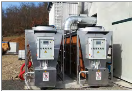
A detail of the dry cooler control panels.
