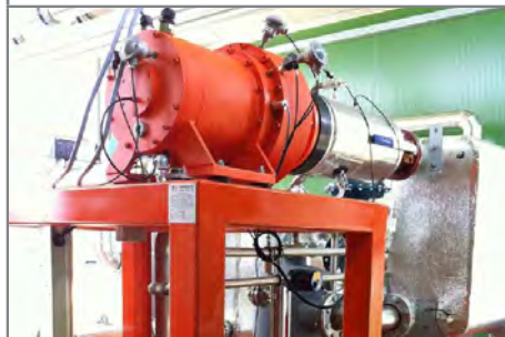
Detail of the 50 kWE turbogenerator
