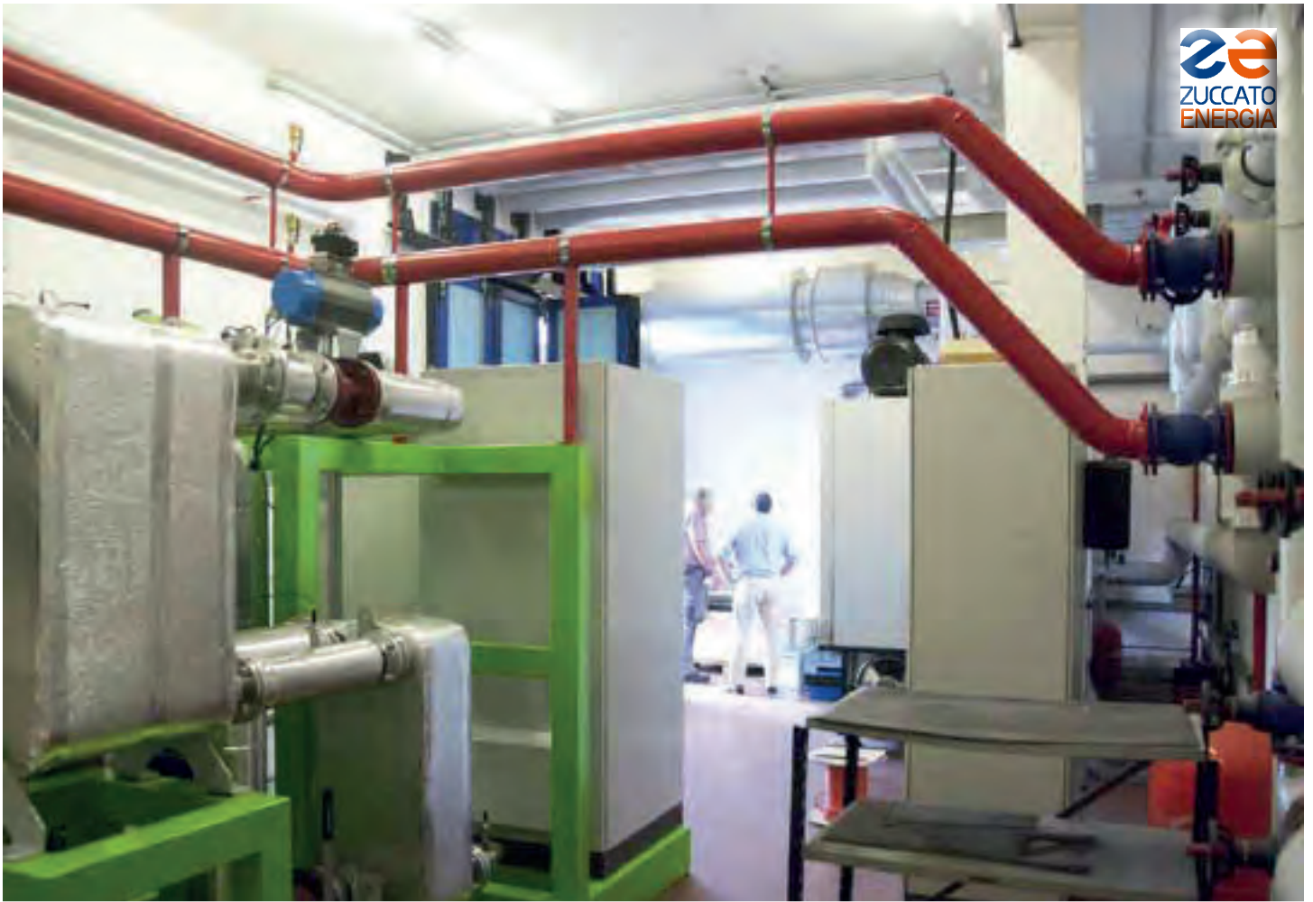
South Tyrol 02 / Bozen: Plant control room as seen from inside.
