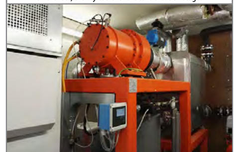
The ORC ZE-50-ULH skid in place inside the building.
