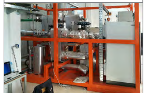
The ZE-60-DSG ORC Module during commissioning
