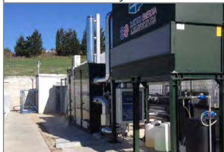
Behind the cooling tower, the ORC module, in its weatherproof containerized enclosure
