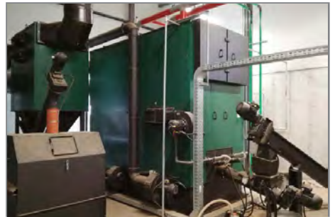
The boiler seen from the right side.
