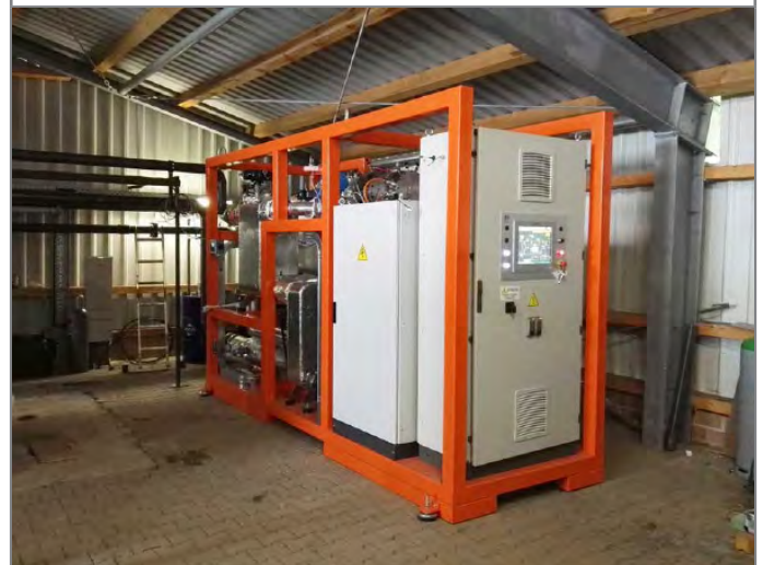
The ZE-40-ULH ORC module seen from the control panel side
