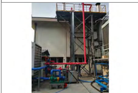
The hot-side piping conveying heat to the ORC. The heat exchanger is on the platform at the top
