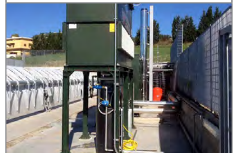
The rear of the tower; in background, the boiler, protected by grid fences, and located under a lean-to
