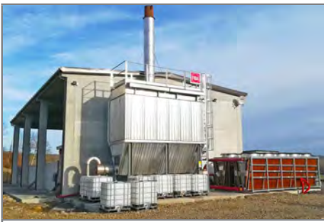
Flue gas treatment system and chimney. On the right, the dry cooler.
