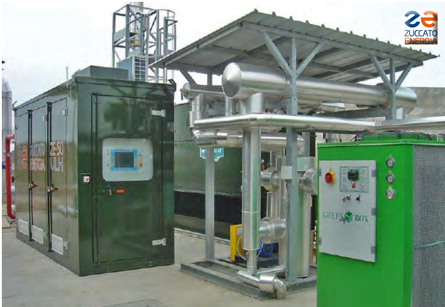
Veneto 01 / Venice: The ORC module in its weatherproof container (left) and the cooling tower (right)
