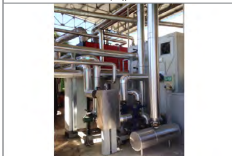
Detail of thermal connections to the boiler, fully insulated
