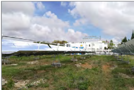
A general overview of the plant
