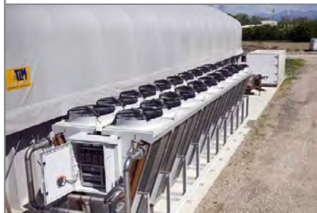
General view of the dry cooler
