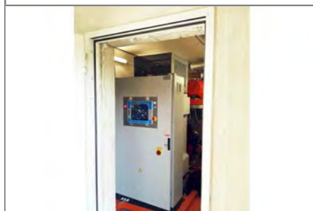
The skid seen from the access door
