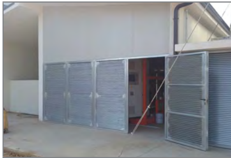
A detail of the ORC building. The skid may be glimpsed through the open door
