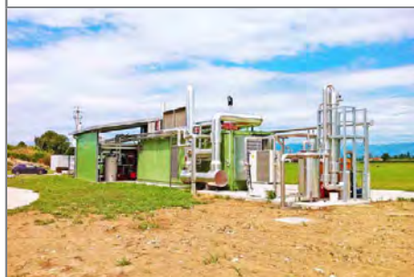
The skid in place under its protective canopy
