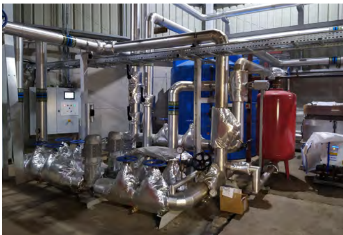
Boiler preheating system and superheated water at the ORC.
