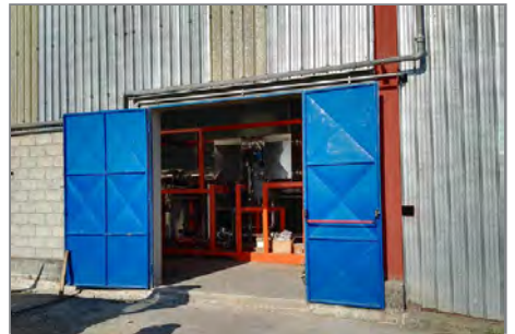
The ORC module skid seen through the shack doors
