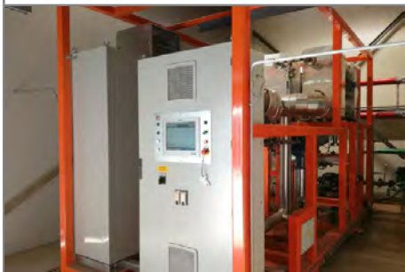
The ZE-150-LT ORC module in place, seen from the control panel side.
