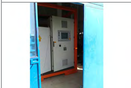
The ZE-60-DSG skid seen from the door
