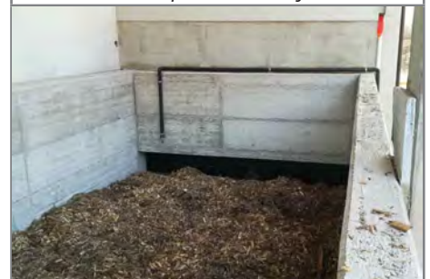
The fuel loading hopper, with feeding rakes on the bottom.
