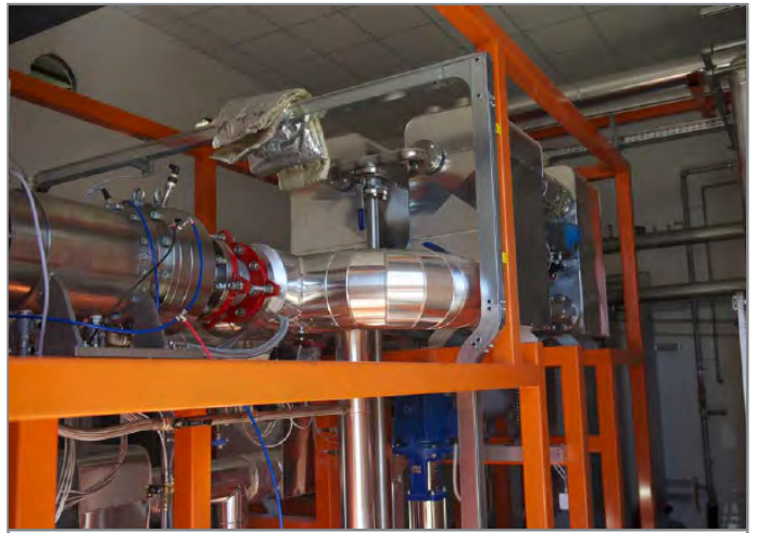
The ORC ZE-150-LT system in detail with the turbine in the foreground
