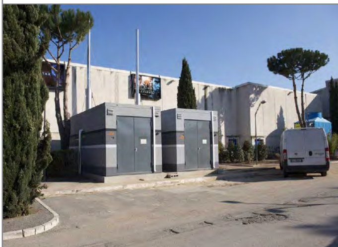
The cogenerators and the cooling tower (blue, right)
