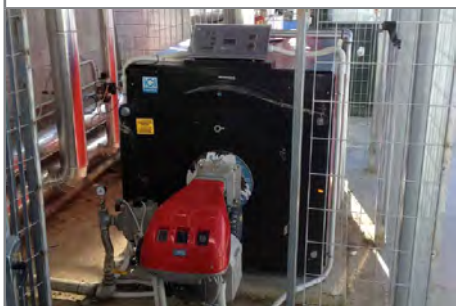
The ICI boiler which supplies most of the thermal energy for the plant.
