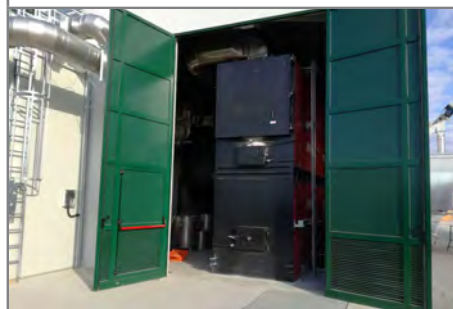
The boiler in its room behind the ORC modules.
