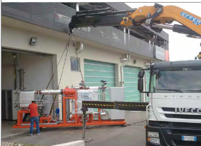
One of the two customized ZE-50-ULH modules is unloaded from the truck
