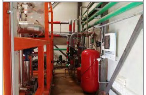
The skid seen from the hydraulic connections side.
