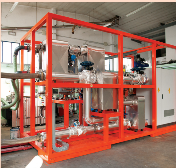
Fig. 3 Zuccato Energia ORC System in Area Test
