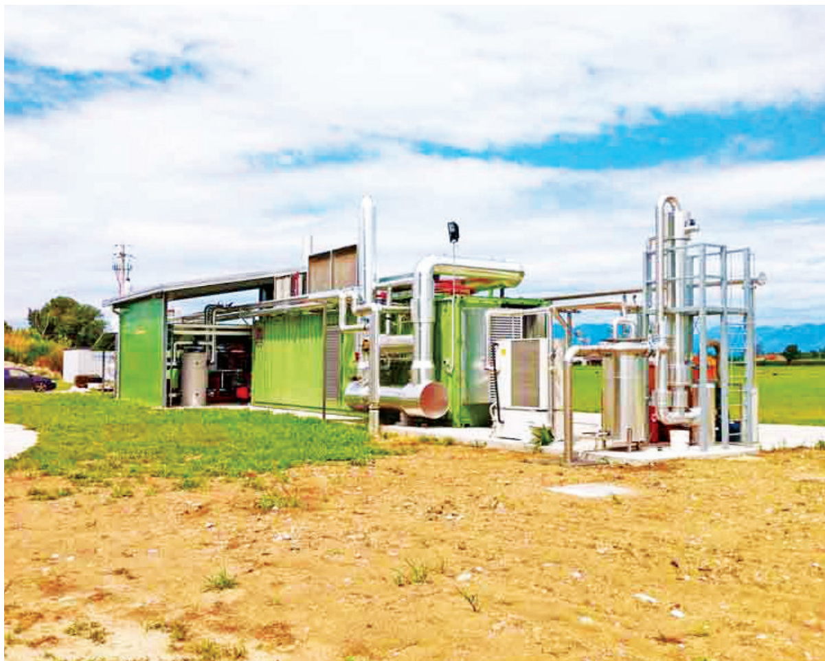
Fig. 2 ORC System in a customer plant
