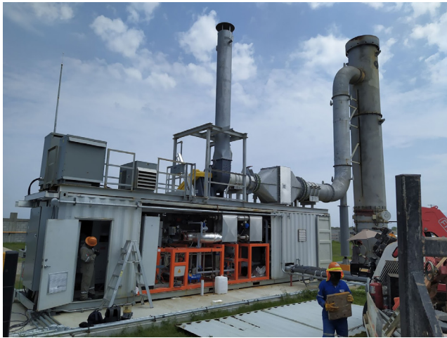
ORC entire installation
